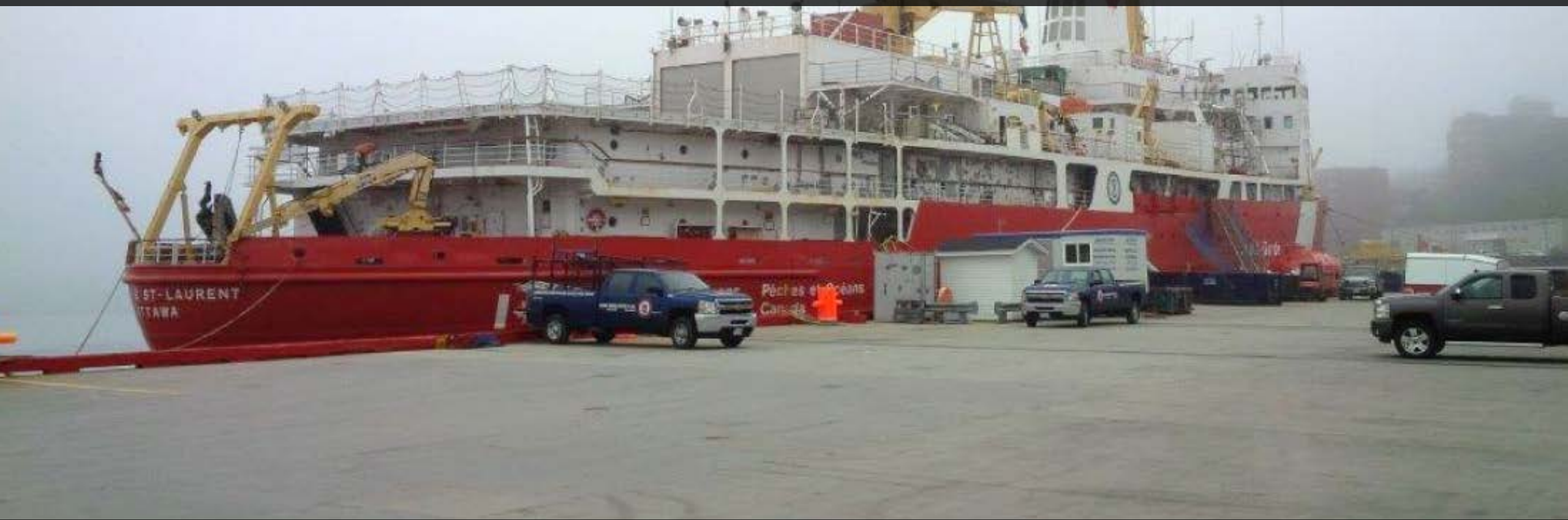
The CCGS Louis S. St. Laurent undergoing alongside repair work by a mobile Heddle repair team
